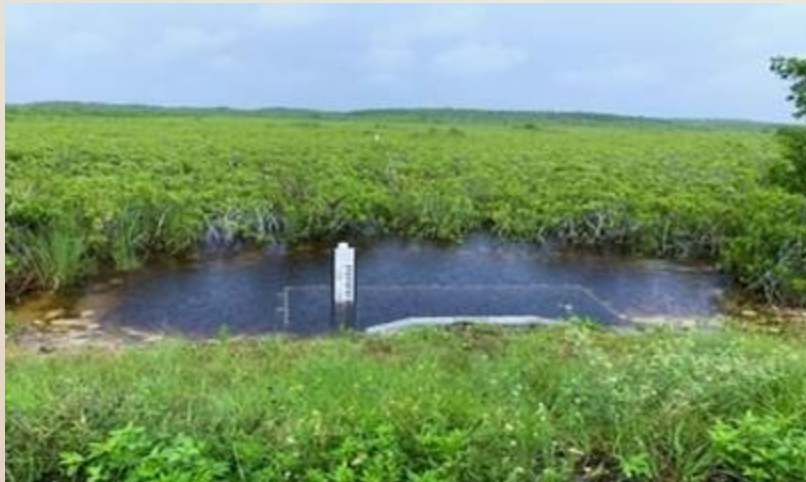
L-31E Flow way culvert providing redistributed freshwater to the coastal wetlands and Biscayne Bay
