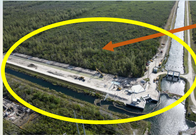
Kiewit Biscayne Bay Coastal Wetlands Phase I Project L-31 Flow-Way, Contract 5B (A) Phase 1 Project Pump Station S-703; Recreational Sites Miami-Dade County Florida Print #240325221 Date: 03/25/24 Lat/Lon: 25.519605 -80.346775 Order No. 75589 Aerial Photography, Inc. 954-568-0444
