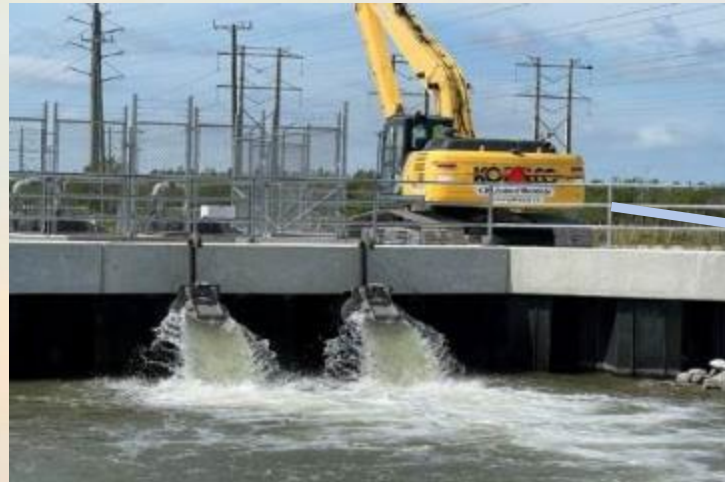
Pump Station S-709
